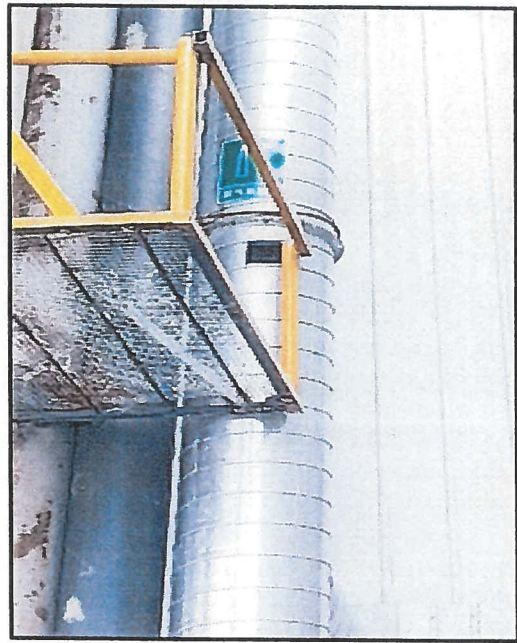
废气排放口标示
